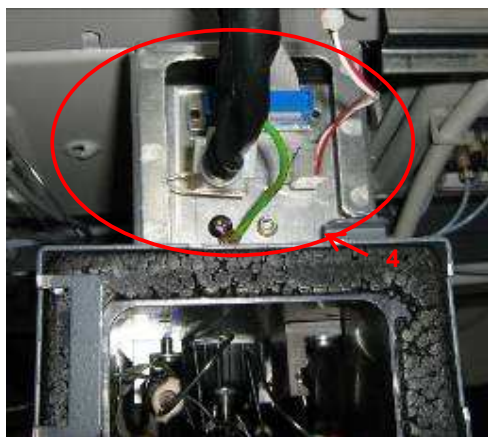
Figure 5: Electrical looms connected to the column oven
