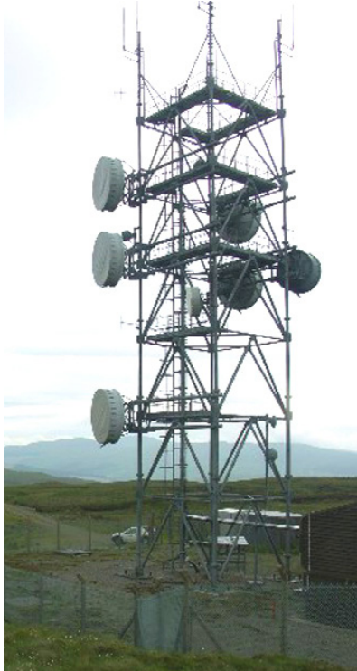
Figure 6a. Microwave repeater showing multiple co-located antennas.[3]
