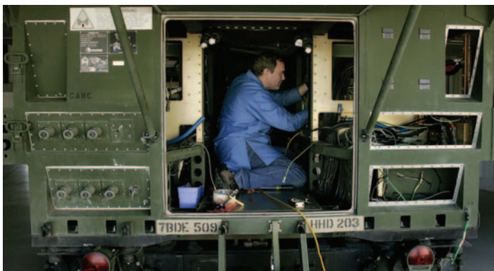
Ralph Werner rewires one of the original Phoenix systems that were sent to Iraq at the L-3 Communications plant. The system is part of a ground satellite dish system that communicates in the field with satellites. (AP Photo/Douglas C. Pizac)
