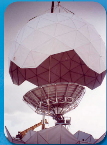
Typical 48-ft (14.7m) diameter MSF radome installation
