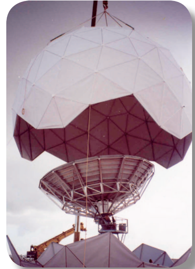
Typical 48-ft. (14.7m) diameter MSF radome installation.
