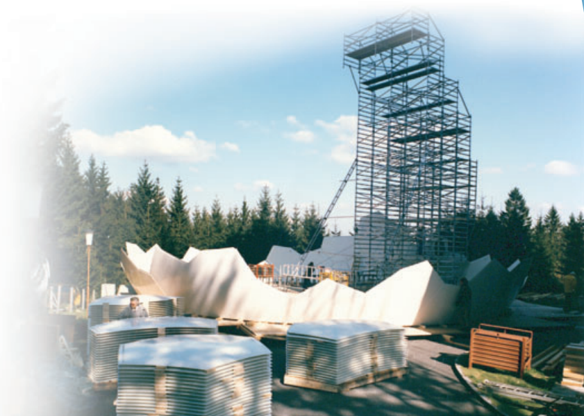
Typical sandwich radome installation
